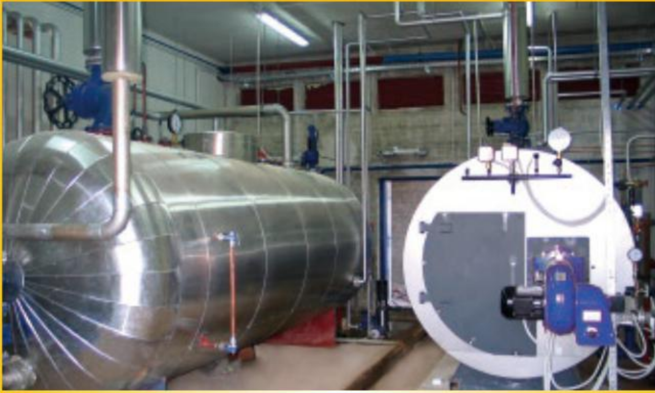
● Steam Boiler & Steam Accumulator
