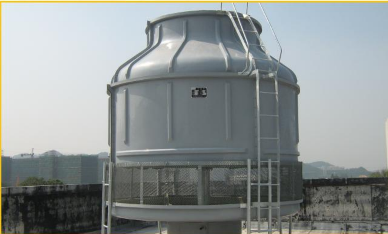
● Cooling Water Tower
